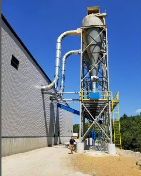
The cyclones rise 62 feet above the concrete foundations. The cyclones use vacuum pressure to draw the sawdust away from the indoor facility, then drop it onto the blue conveyor system where it heads back inside for packaging.
